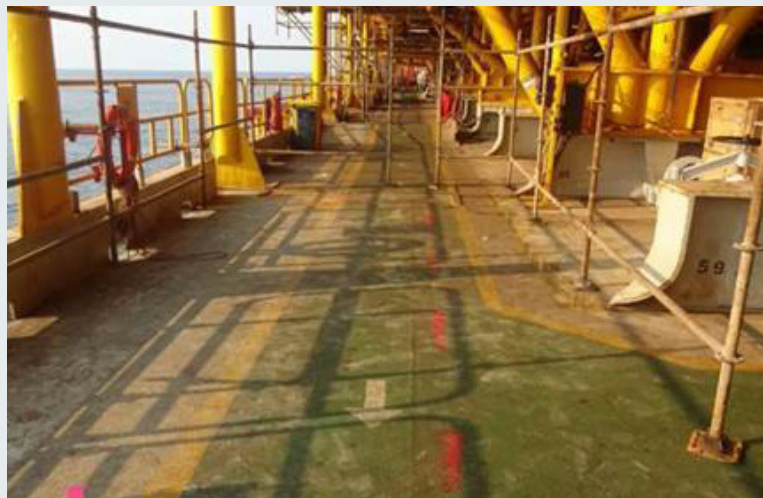
Figure 4: Corroded deck plating of an FPSO (Courtesy of Cold Pad)
