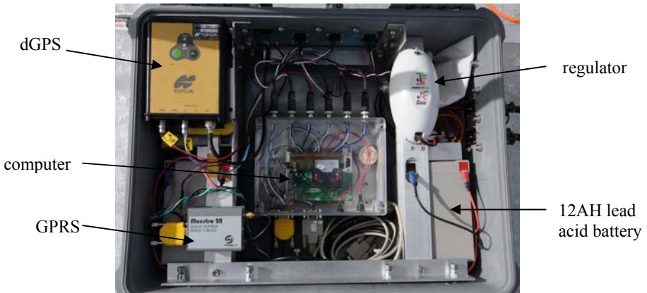
Fig. 3. Base station case showing major components
